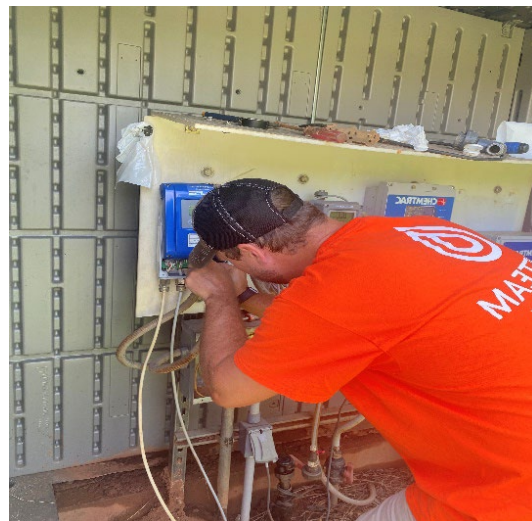
*Pictured right, Clay Stuart installs the new flow meter display. Grounding rods have been installed.
